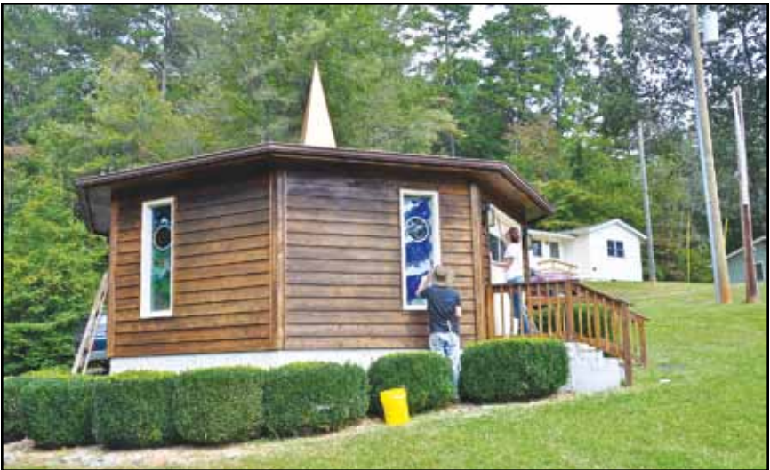
Repainting window casings and doors of the Shrine of All Faiths Meditation Temple at CSA headquarters. September 2013
