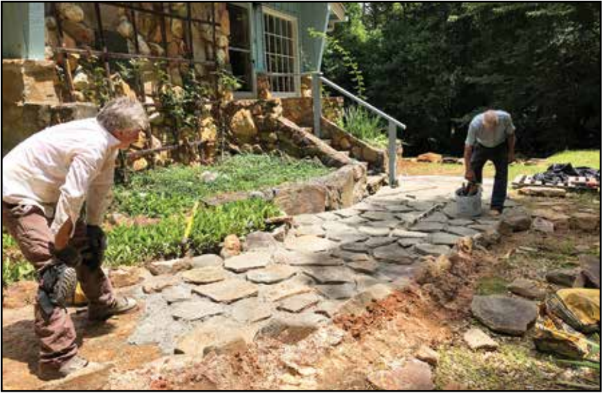
Above: Rodney Amig and Rob Callaway, longtime CSA employees, laying the foundation for a new, safer sidewalk at a CSA guest house. – July 2020
